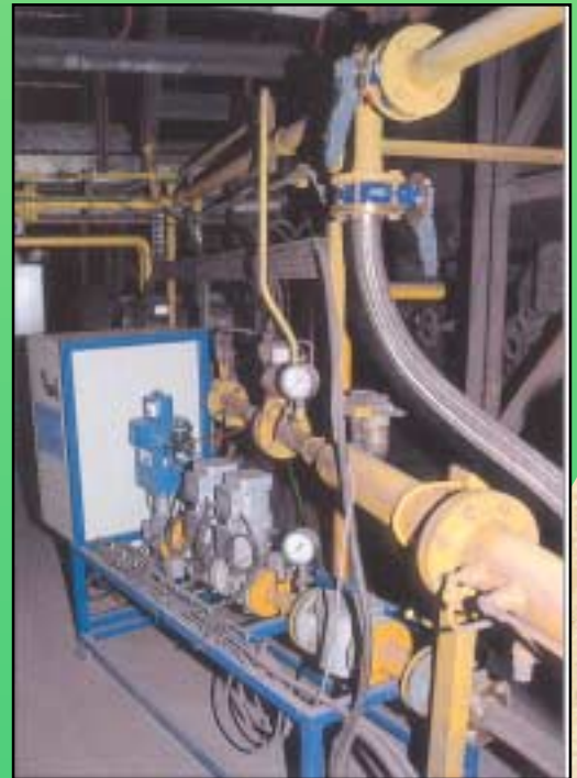
New gas pipe
